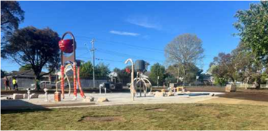
Progress at the Brown Hill Splash Park site. Image supplied by the City of Ballarat
